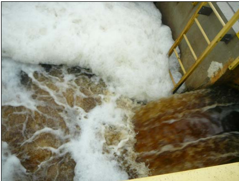
Illustration 14: Typical foaming at influent surge box at TC-ATS facility.
