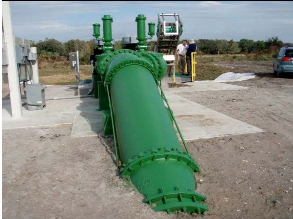
Illustration 2: Image of the 15-MGD mixed-flow pump station at the TC-ATS.
