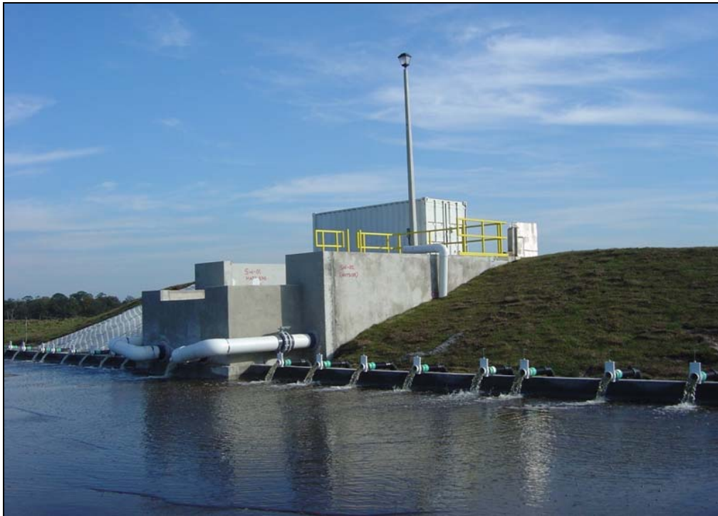
Illustration 3: Image of the TC-ATS inflow surge, distribution manifold and laterals and monitoring station.
