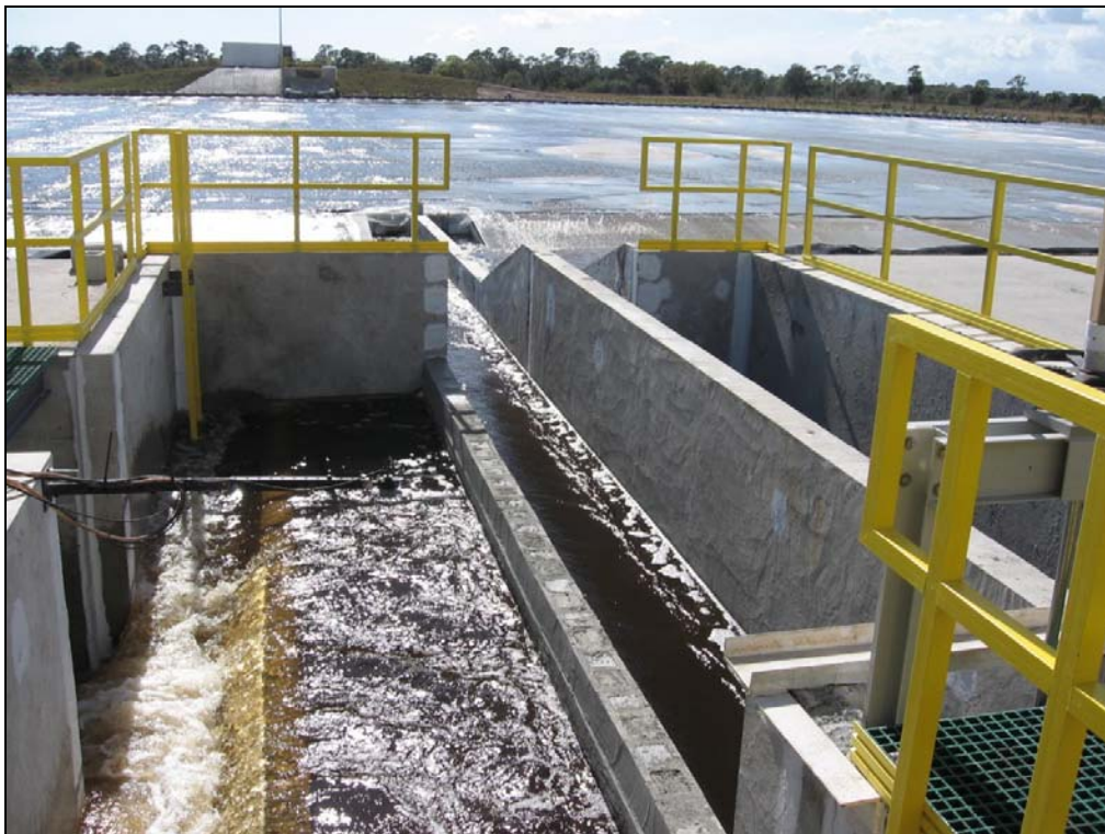
Illustration 4: Image of the TC-ATS outflow and first stage solids recovery unit.
